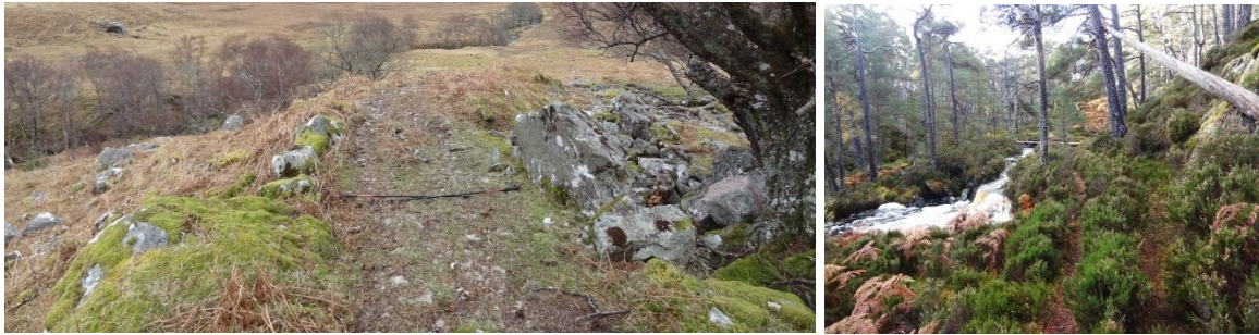
These paths in Glen Elchaig and Strathfarrar (SP9.04 / 35) have rare cuts through boulders or bedrock ledges where a six-foot width is verifiable.
